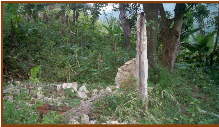
Home destroyed by Hurricane Matthew
